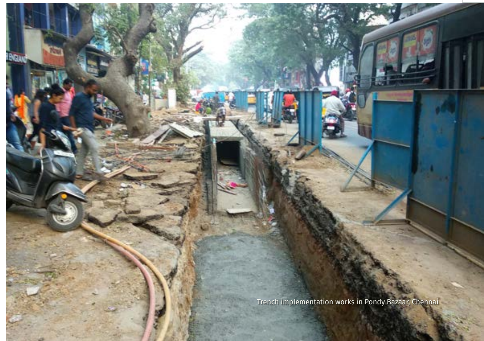
Ducts in DP Road, Pune
